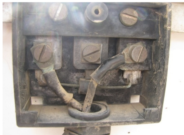
Fig. 8.18: Corrosion in output terminals
