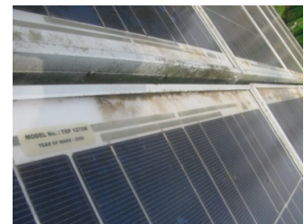
Corrosion & Algae growth on frame
