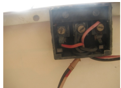
Corrosion in output terminals
