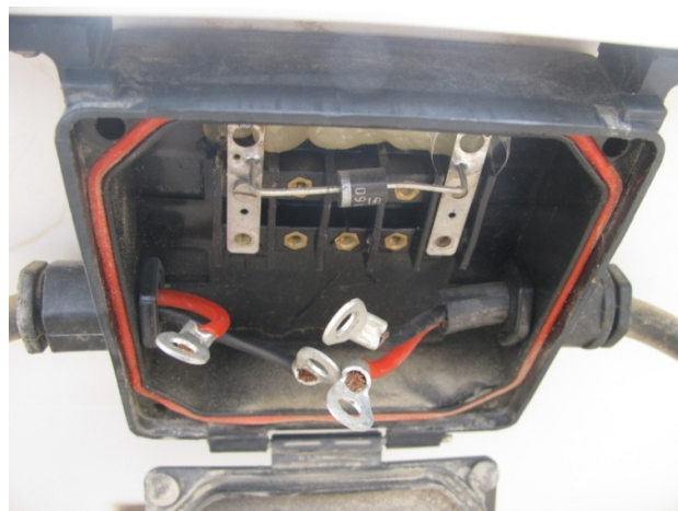
Fig. 8.28: Junction box with good sealing, which has prevented corrosion of output terminals and Bypass Diodes
