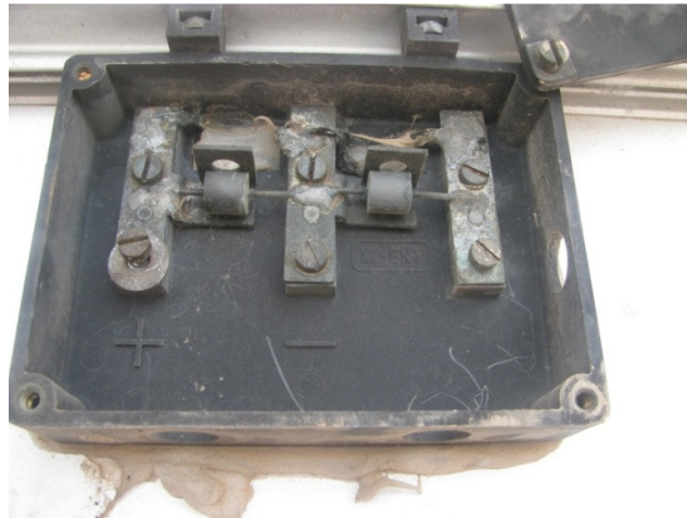
Fig. 8.27: Junction box with no sealing, which has lead to corrosion of output terminals and Bypass Diodes
