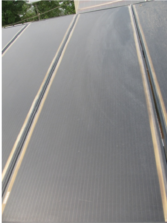
Fig. 8.35: 13 years old CIGS Module installed in Composite climate
