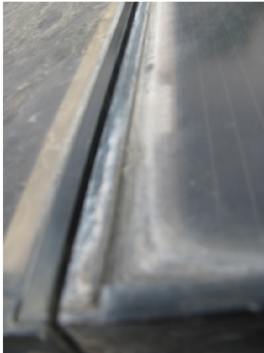
Fig. 8.38: White deposits (salts) at the edges of the CIGS Module
