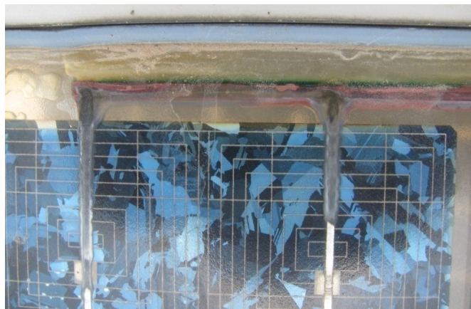
Fig. 8.17: Corrosion (seen as red, green & black discoloration) in the string interconnect of a PV module installed in Hot & Dry zone in 1988.
